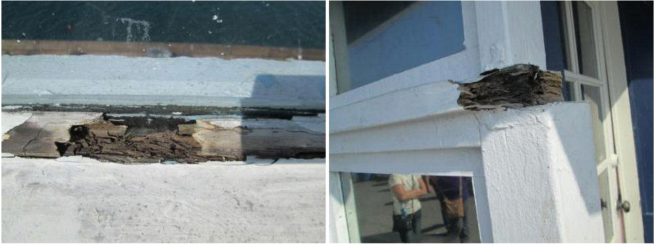
View of rotten trim
