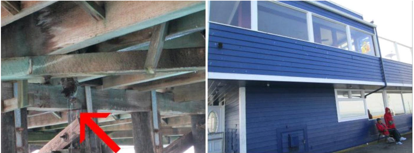
View of leak area under building
