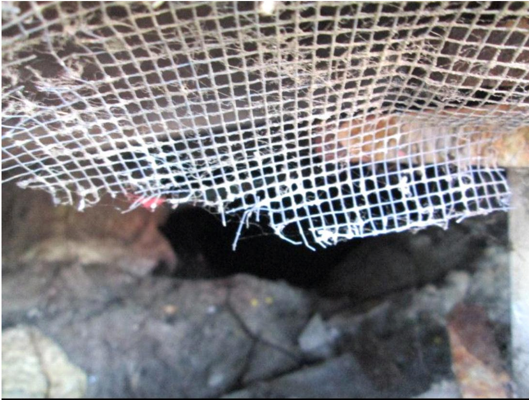
broken vent screen
