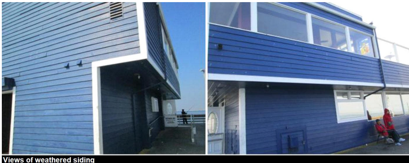
Views of weathered siding
