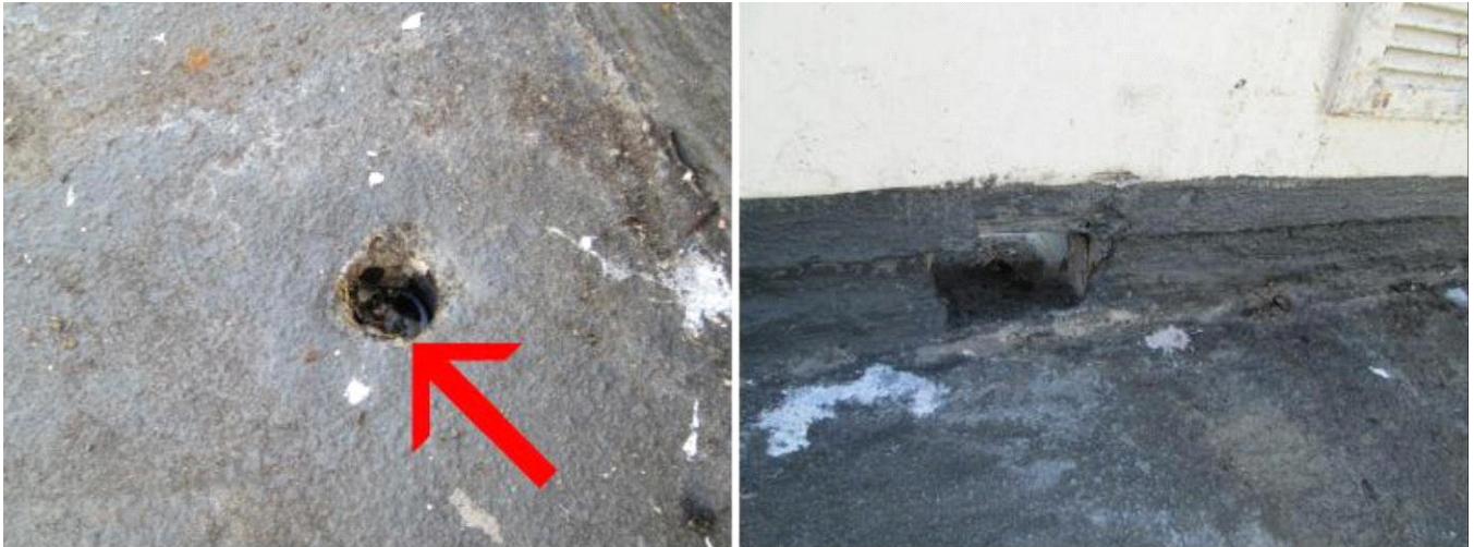
Deck drain is clogged & full water
