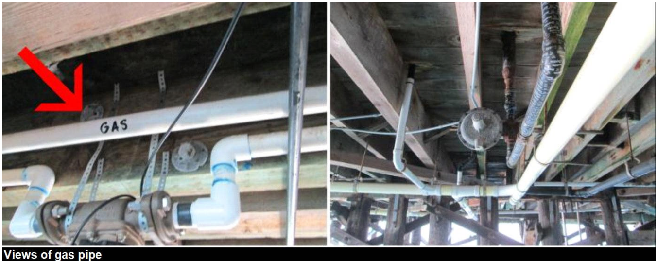
Views of gas pipe
