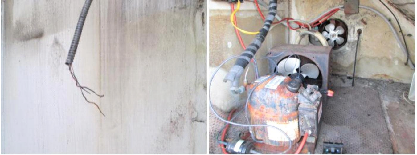
Exposed wiring in areas
