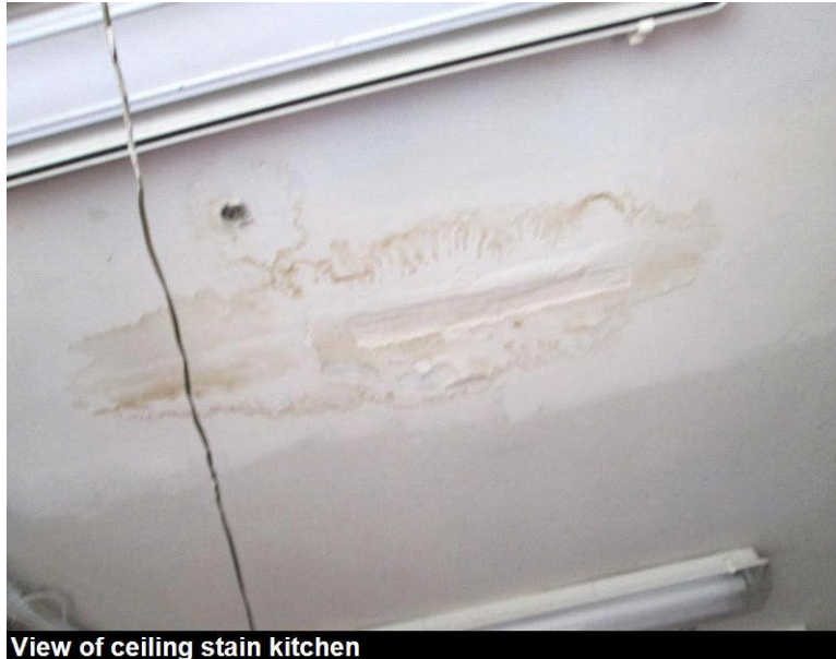
View of ceiling stain kitchen
