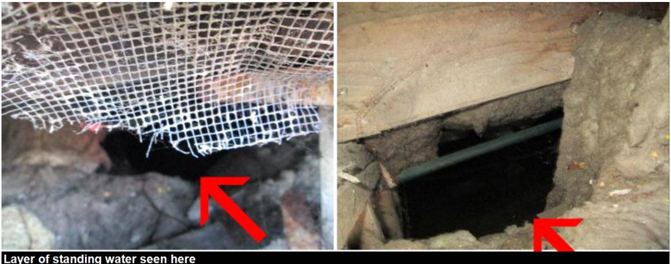
Layer of standing water seen here
