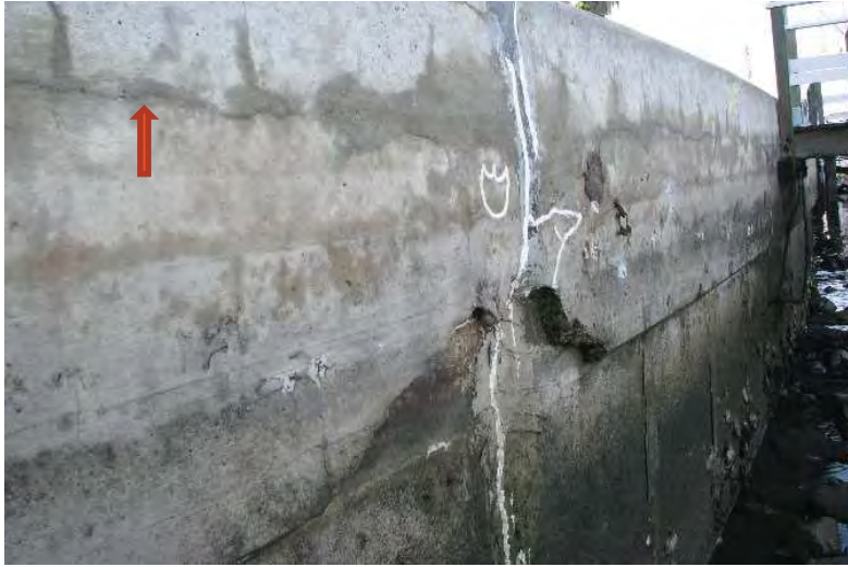
Figure 4 - Cold joint visible along Coping Type D
