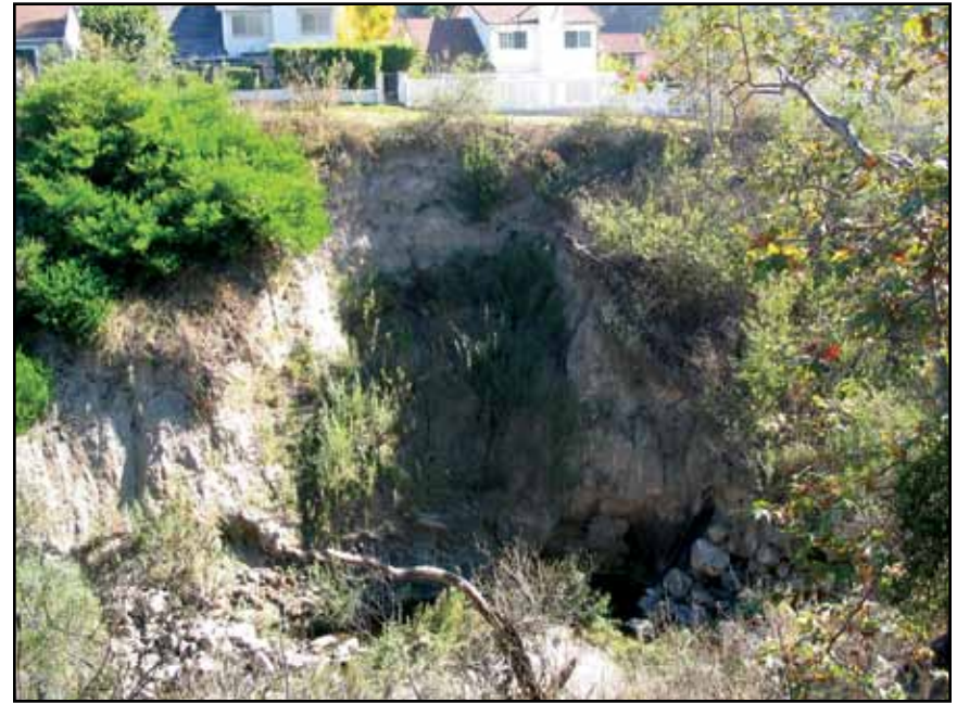
Figure 10.8 Erosion in Serrano Creek
