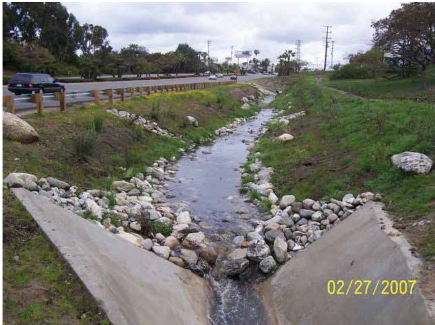
Figure 5.3 Newport Boulevard bioswale.
