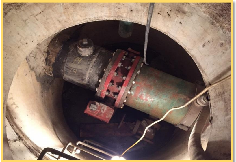
18-inch Distribution Valve
