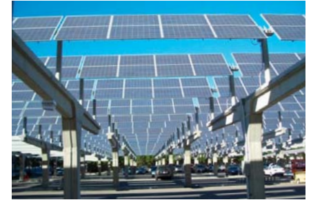
PV Arrays as Parking Lot Shading
