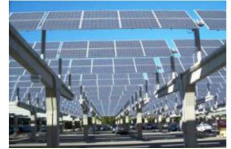
PV Arrays as Parking Lot Shading
