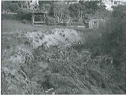
West Side Bank Erosion
