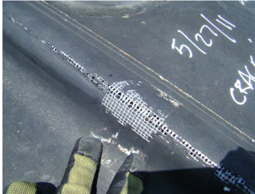
BCR RPP exposed scrim reinforcement
