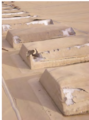
RRP walkway float material failures, Marion Co., OR - 2008
