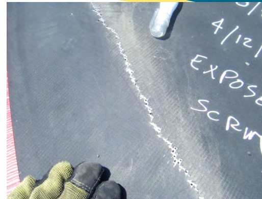
BCR RPP exposed scrim reinforcement
