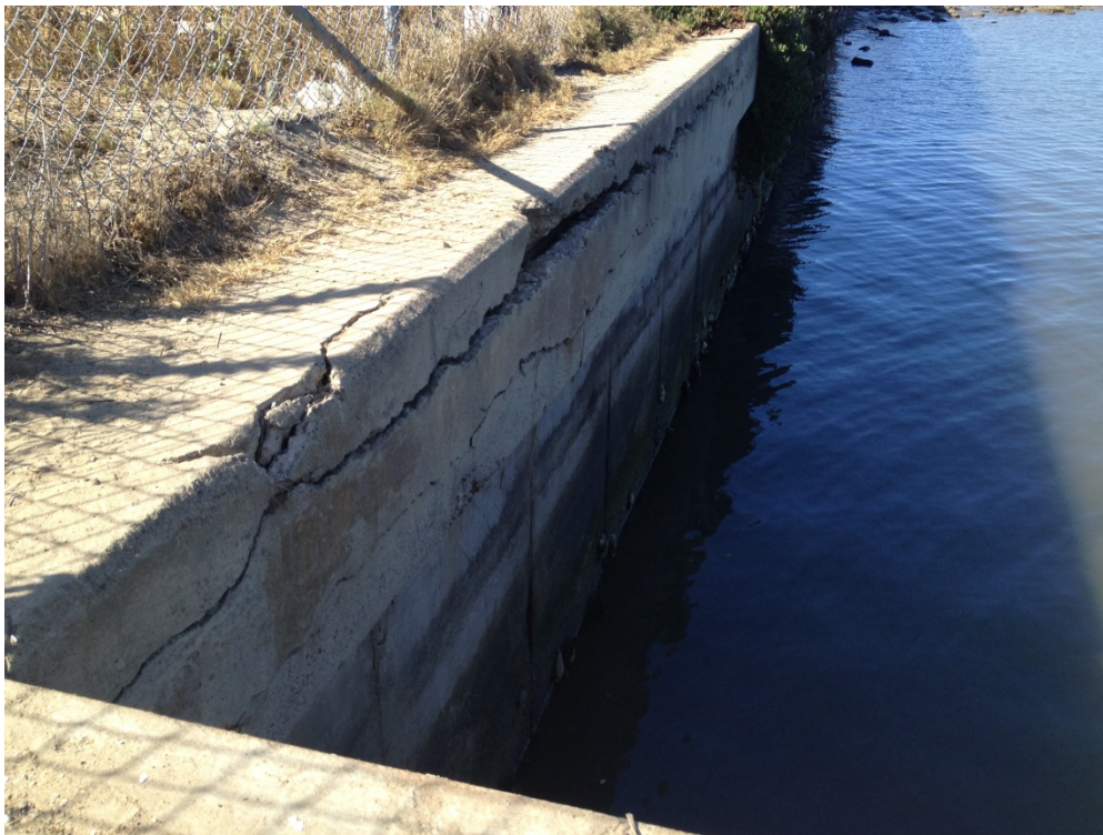
Photograph 2. Cracking in wall cap.
