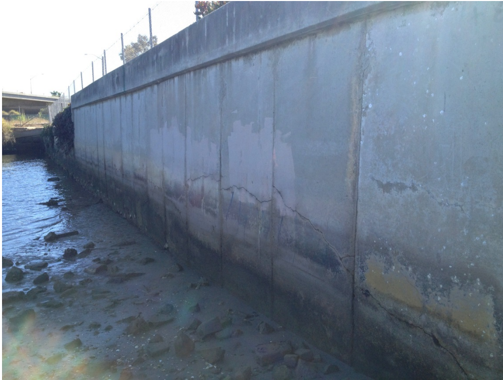
Photograph 1. Northern stretch of wall, showing horizontal cracking on the face.
