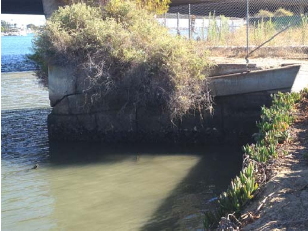
Photograph 3. Spalling and cracking at wall outer corner.
