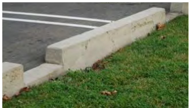
Stormwater Curb Treatment
