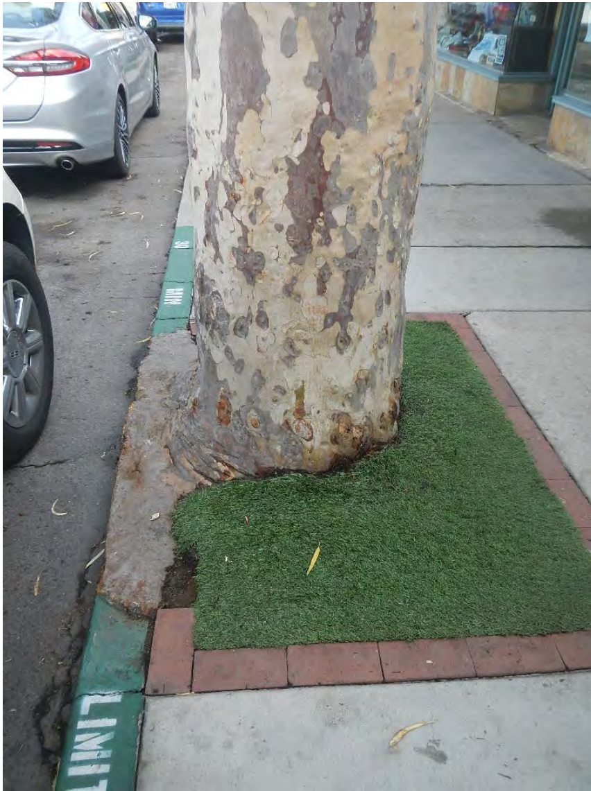
#8 red gum growing over the curb to spread the load, at 210 Marine
