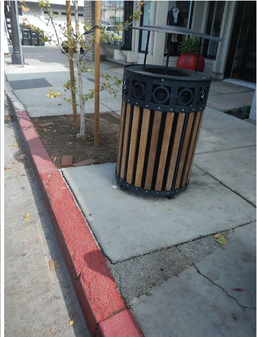
Note lifted sidewalk even after new tree is planted.
