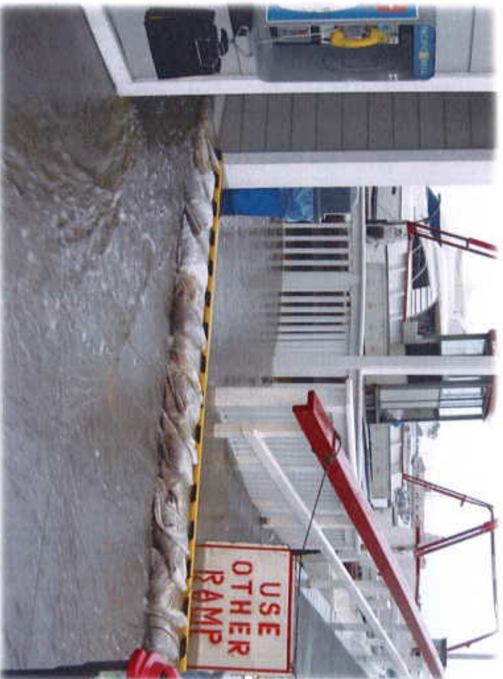
Seawall Gap – Ferry Landing
