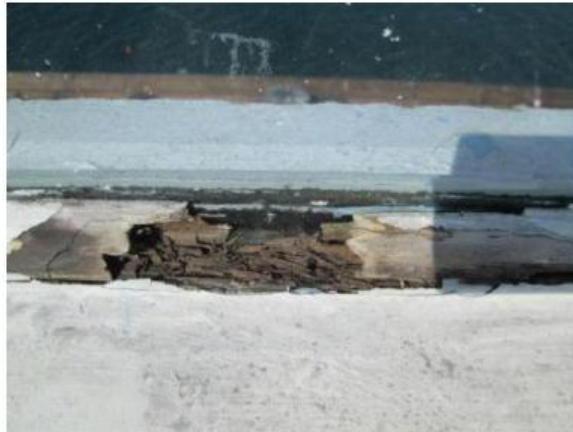
View of rotten trim
