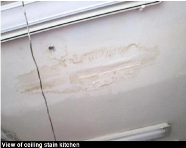
View of ceiling stain kitchen
