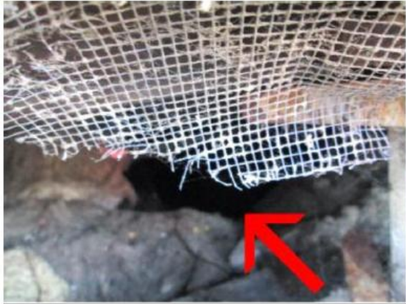
Layer of standing water seen here
