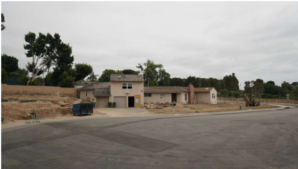
IMAGE 2 GARAGE ON SUBJECT PROPERTY GRADED SUBSTANTIALLY LOWER THAN ADJACENT LOT
